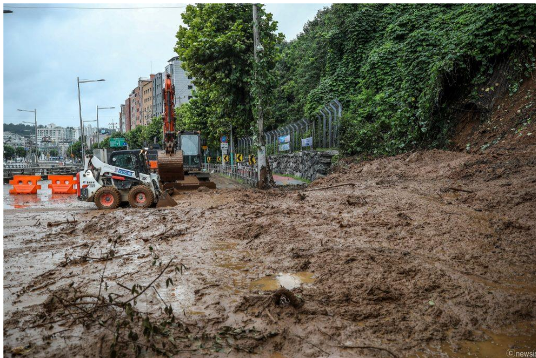
Flood damage in Seoul, South Korea, August 2022. Photo: Government of Seoul
